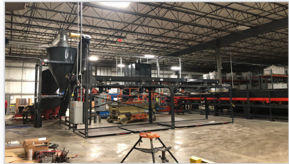
The Wilmington plant's grinder can process up to 7,000 pounds of plastics per hour
